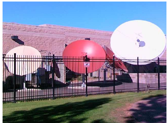
RIVA Earth Station Antenna Farm
