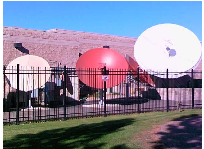
RIVA Earth Station Antenna Farm
